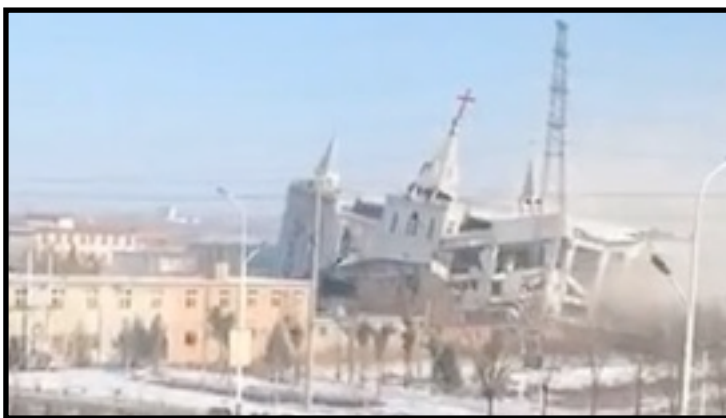
Screen grab of footage of the demolition of Golden Lampstand Church in Linfen city in northern Shanxi Province, Jan. 9, 2018.
